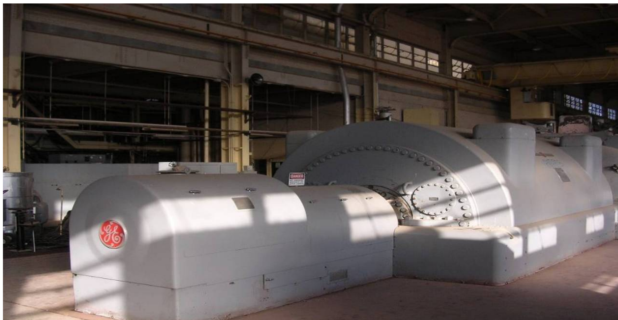
Paint Creek Plant - Turbine & Genrator Sets - Bid#09-340-66.doc
